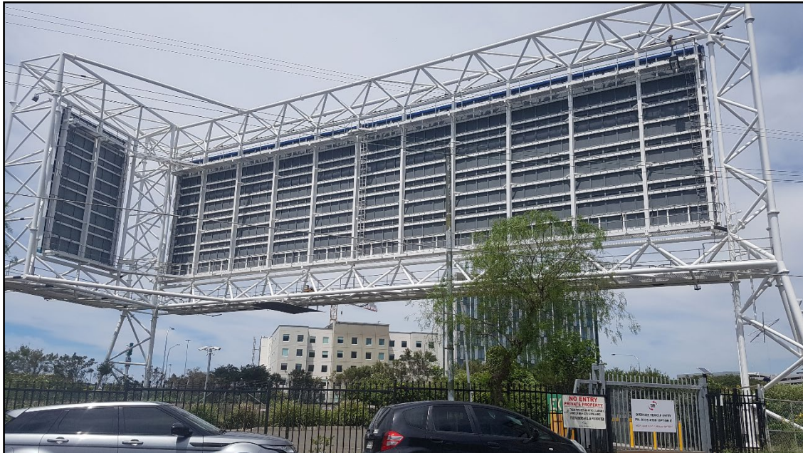
Figure 14: View of the vehicular entrance and advertising sign structure at proposed Site A (western lot) to the west of the subject site
